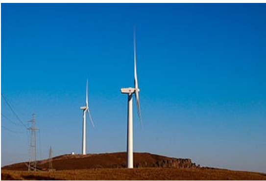
Figure 7: Onshore Horizontal Axis Wind Turbines in Zhangjiakou, China
